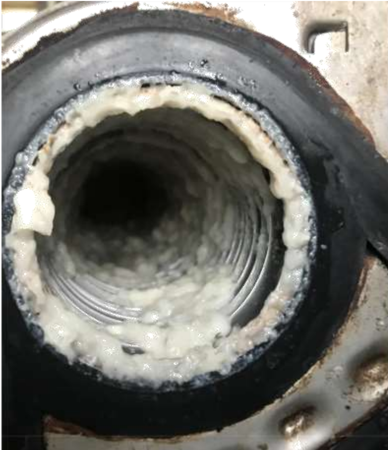
Deposits found in the pipe
