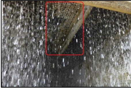
Plugged fills restricting water flow prior to HydroFLOW
