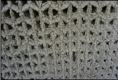
Rock hard scale on drift eliminators prior to HydroFLOW
