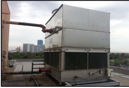
Cooling tower prior to the HydroFLOW installation
