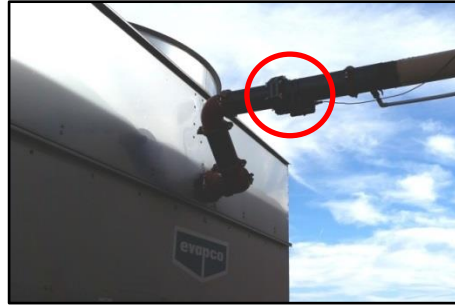
Installed HydroFLOW device
